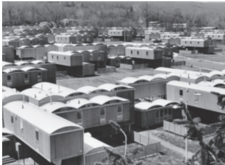
Paul Rudolph, Oriental Masonic Gardens under construction, 1968-1971. New Haven, Connecticut. Courtesy of the Library of Congress.
