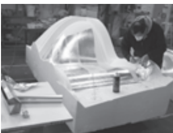
Mold preparation for Bloom House Lantern designed by Greg Lynn Form. Kreysler and Associates used CNC milled foam molds as a form.
