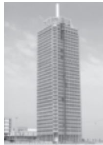
Dubai World Trade Center, construction photograph April 30, 1979, courtesy of Stephen Finch, James Sunley
