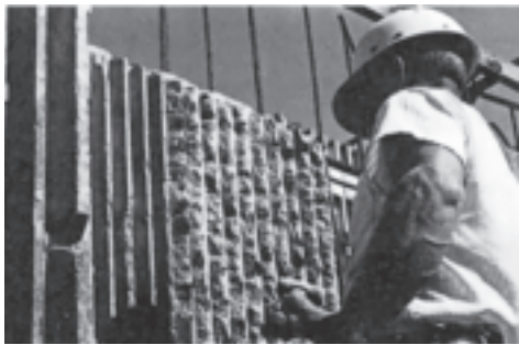
Worker hammering “cordoroy” concrete of the Yale A&A Building, 1963, photograph by Robert Perron
