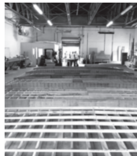
Construction progress of the coastal research station for the Peabody Museum of Natural History on Horse Island, Branford, Connecticut, summer 2020
