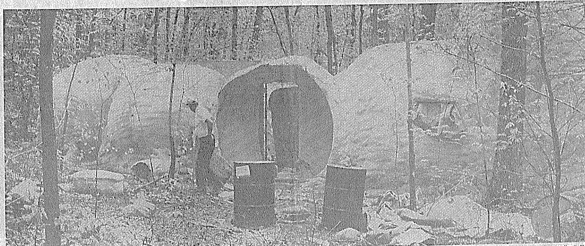
Yale University architecture students built this structure with polyurethane foam sprayed over balloon
